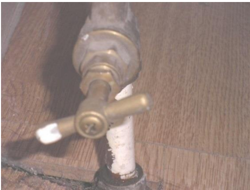
MAIN WATER CUT OFF
