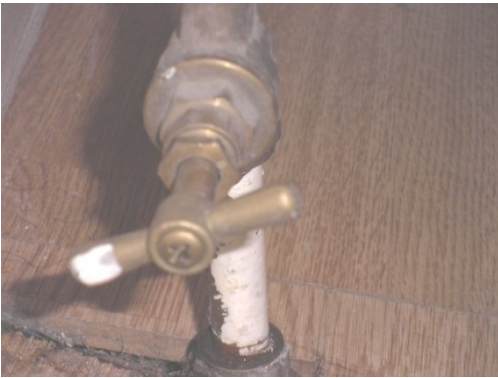
MAIN WATER CUT OFF
